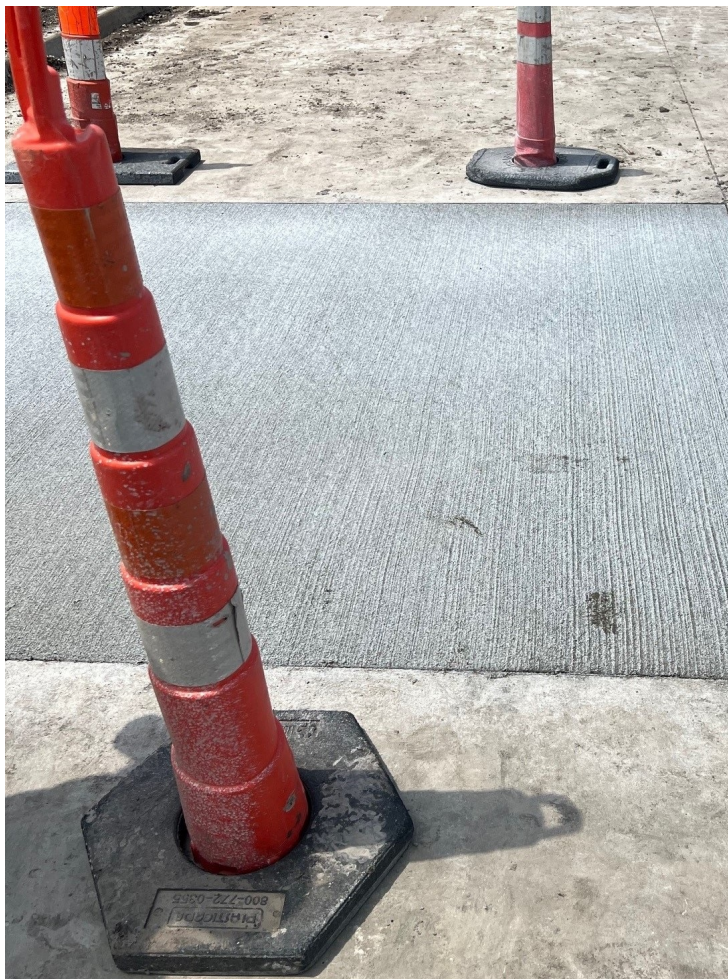
Ineffective curing application
