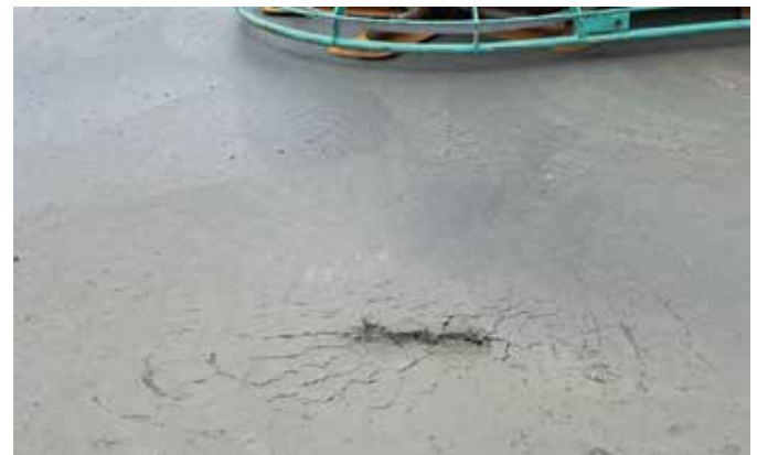
Fig. 2: Surface tearing during troweling
