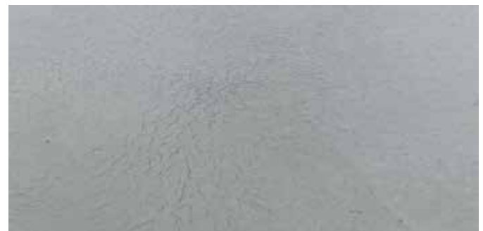
Fig. 3: Surface cracking during troweling operation, concrete below surface is still plastic
