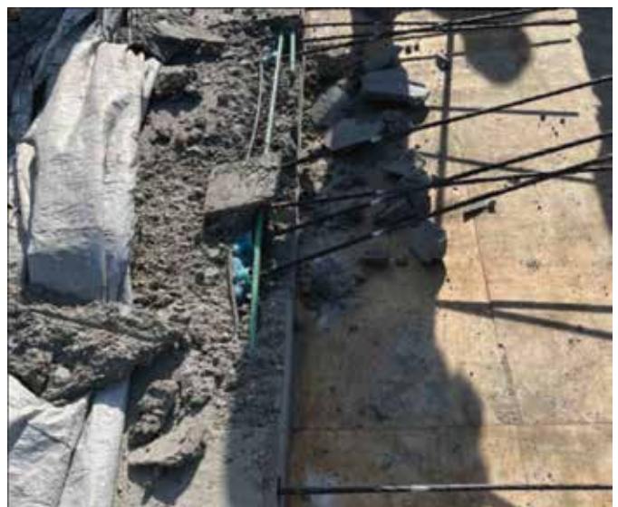
Fig. 12: Tendons in a concrete slab constructed with Type IL concrete were stressed based on a maturity calibration for Type I cement concrete. The strength of the Type IL cement concrete was overestimated, resulting in slab blowouts
