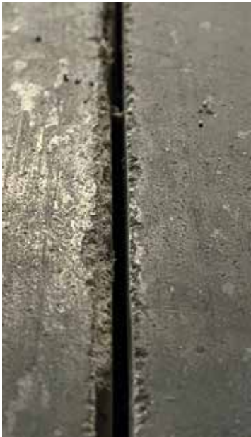
Fig. 9: Saw cutting too early results in raveled joint edges (photo courtesy of Scott Metzger, Metzger/McGuire)
