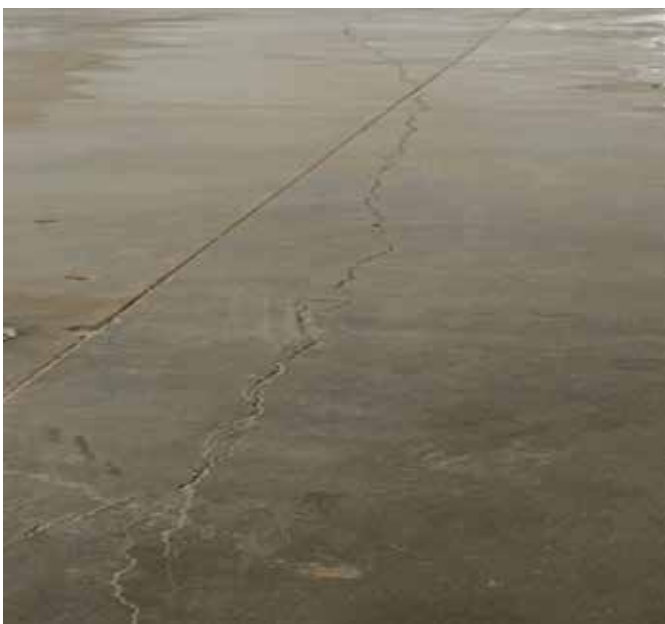
Fig. 10: Saw cutting too late results in cracking (photo courtesy of Scott Metzger, Metzger/McGuire)
